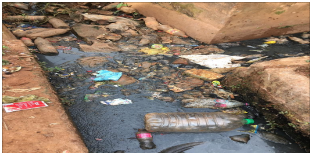
Figure 7: Stagnation of wastewater due to plastic waste
